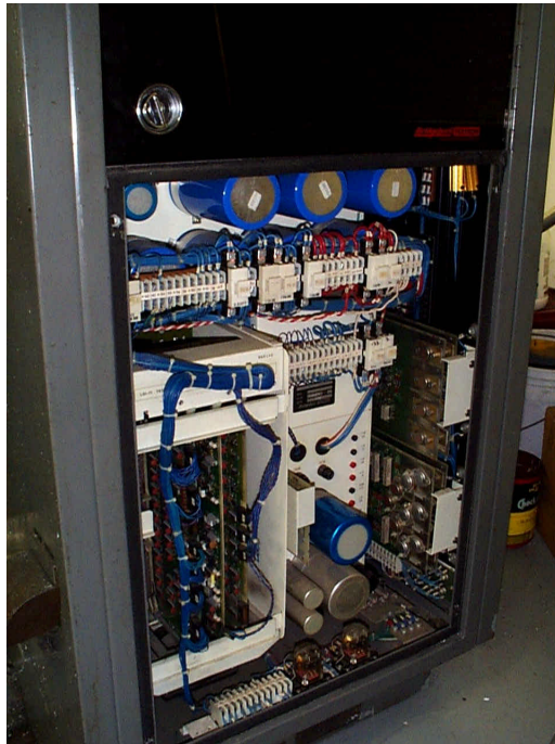
The inside of the BOSS 5 controller cabinet.
