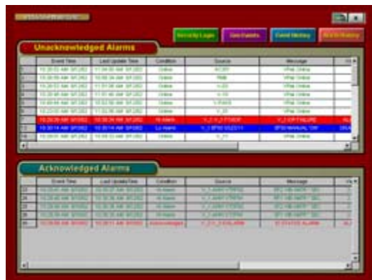
Alarm Monitoring View Screen
