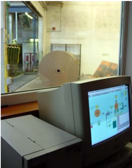
Final Control Room
