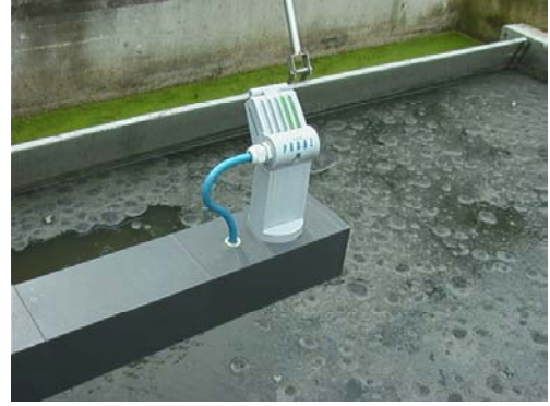
Fig. II.31. Level measurement in sewage-treatment plant.
