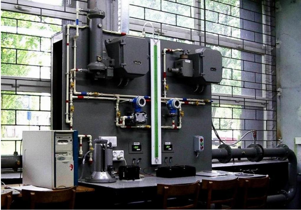
Fig. 70. Overview of the installation for researching of air flowmeters properties.
