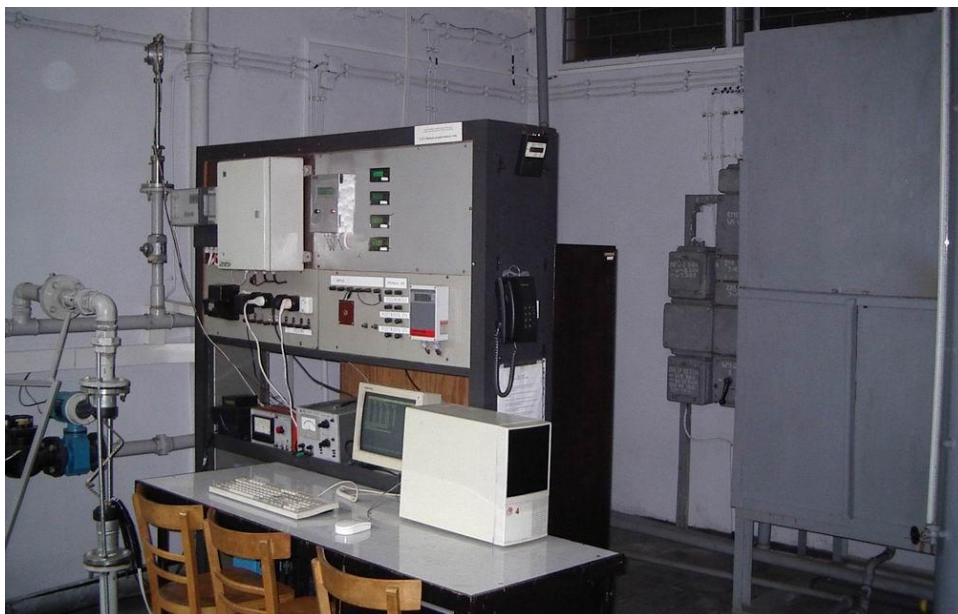
Fig. 69. Overview of the installation for researching of water flowmeters properties.
