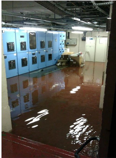
Figure 12.7 Flood at Portland causes outage.
