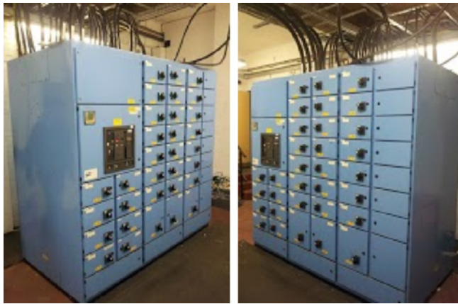
Figure 12.4 Woodhouse building LV switch panel.
