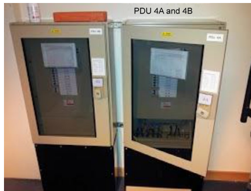
Figure 12.5 Meter installation for servers in the server room.
