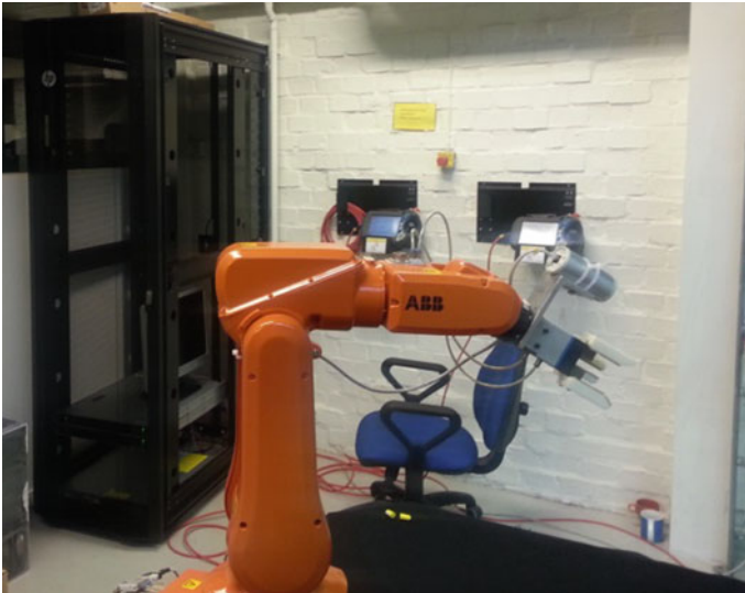
Fig. 10.6 Cloud servers in the black cabinet and an industrial robot
