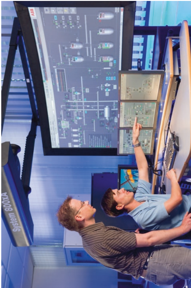
Fig. 11.4 A look at the control center 800xA. (Photo: ABB)
